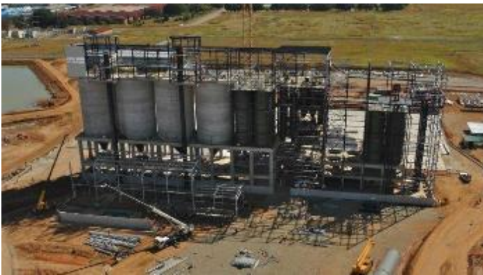
Consol Nigel Batch Plant
