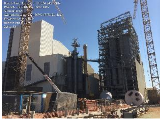
Batch Plant, Johannesburg
