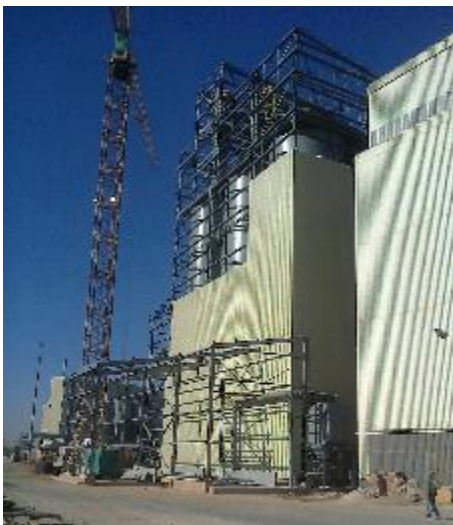
Batch Plant, Johannesburg
